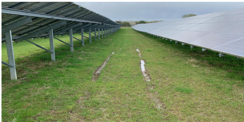
Photo 15.21: Example of Minor Ruts Caused by Vehicles
