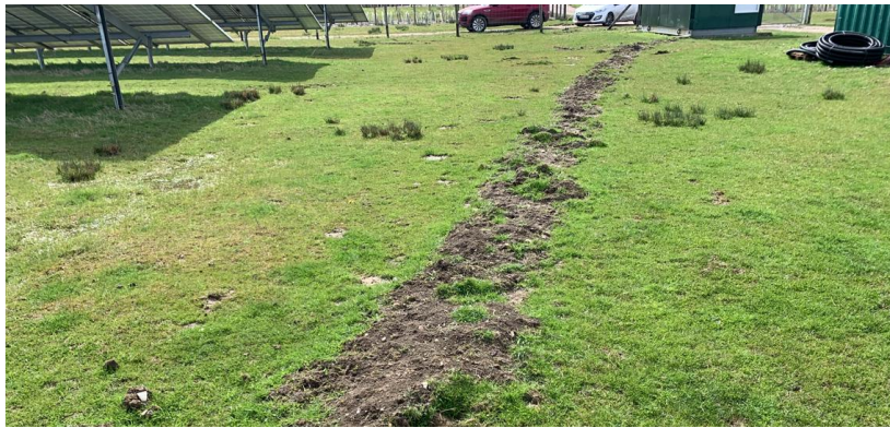
Photo 15.22: Trench During Wet Period
